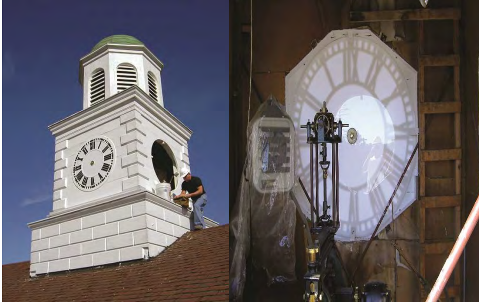
City Hall Clock Tower Face Repair and 1930 Seth Thomas custom made clock inner workings.
